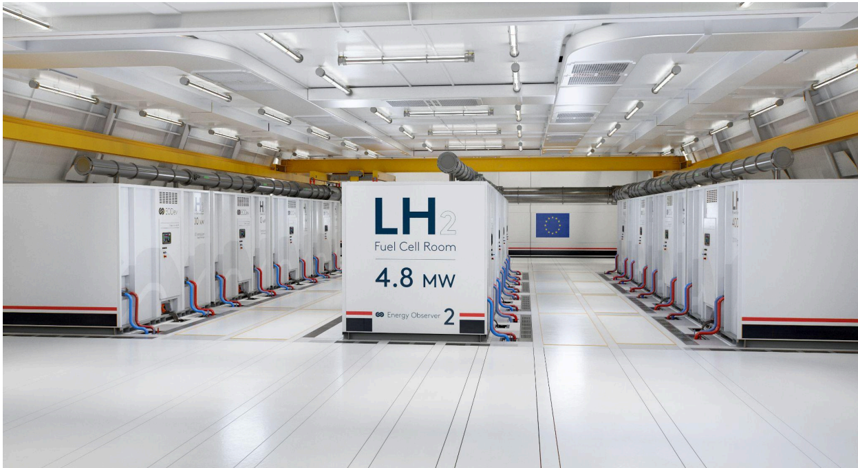
Fuel Cell Room - © Kadeg Boucher
